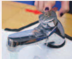
A small amount of water is diverted from the pipe, oozing out at the top
